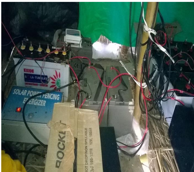
Photo 3.3: Batteries inside the cabin
