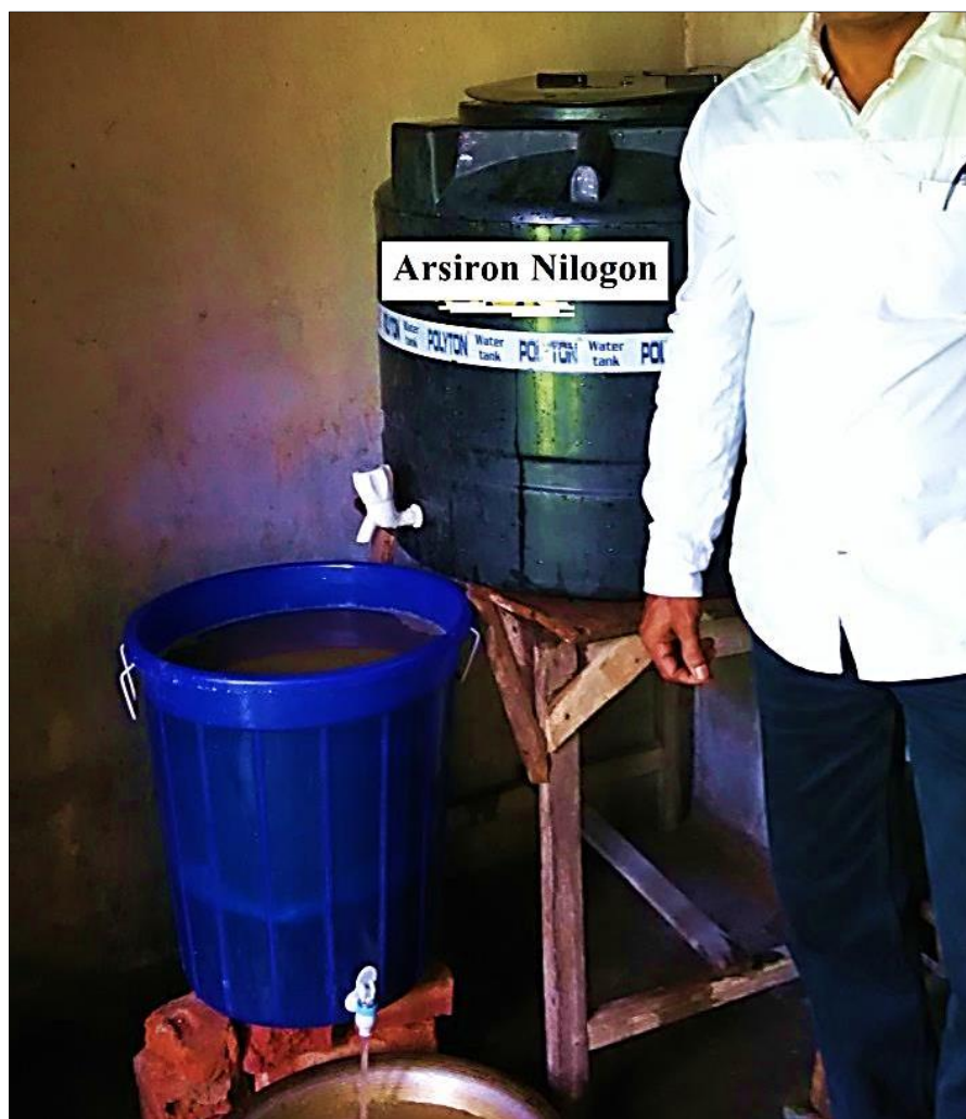
Figure 2.2: One small 200 L community unit installed at Tipomia Bagodia L. P. School, Titabar, Jorhat, Assam.
