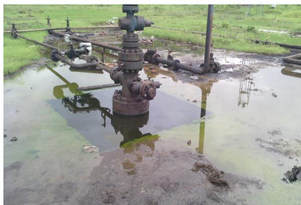
Fig. 2.3.: An oil contaminated drilling site in Borhola Cluster 1
