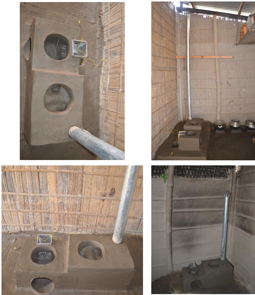
Fig. 4.6 TIFICS installation at selected households
