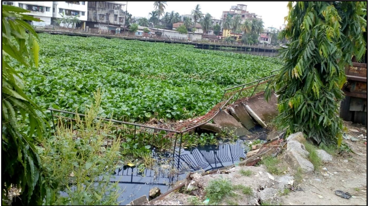
Figure 5.11: Broken sidewalk and growth of water hyacinth due to lack of maintenance
