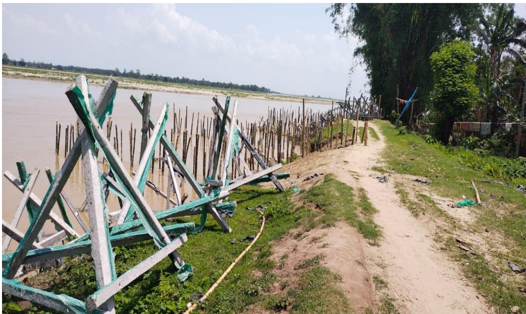
Image 5.2 Porcupine as an hydraulic infrastructure to control the shifting landscape before floods. Image was taken on 18 th December, 2021
