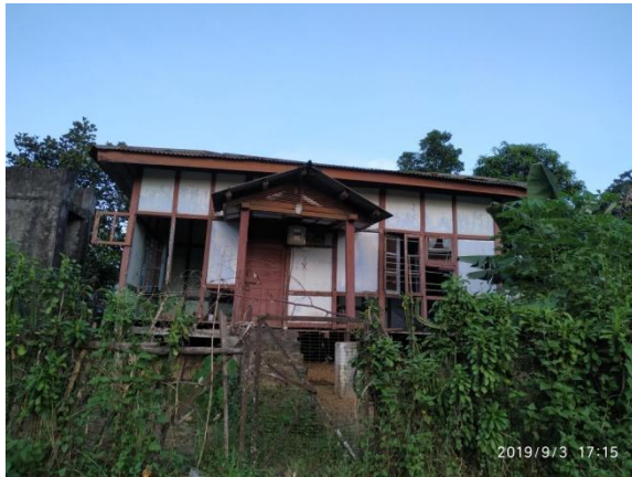
Figure 4.4. Dilapidated Quarter 2 Source: Author
