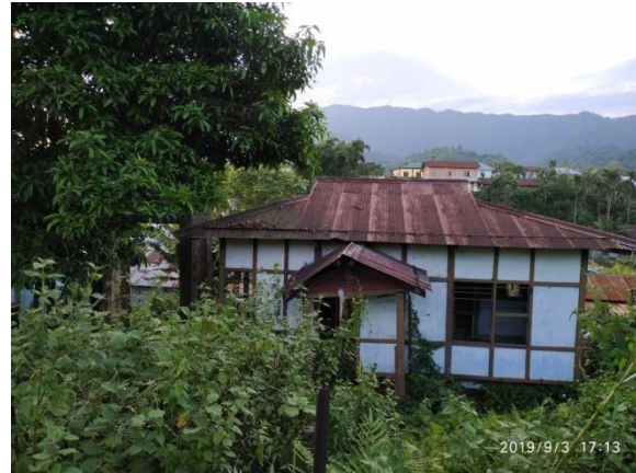
Figure 4.3. Dilapidated Quarter 1 Source: Author
