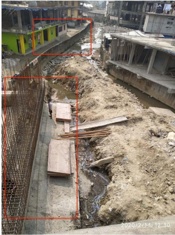
Figure 5.5. River-bed encroachment by people and bridge construction by the State.
