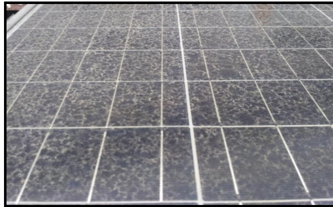
Figure 3.17 The photograph of the horizontally placed PV modules under the soiling.
