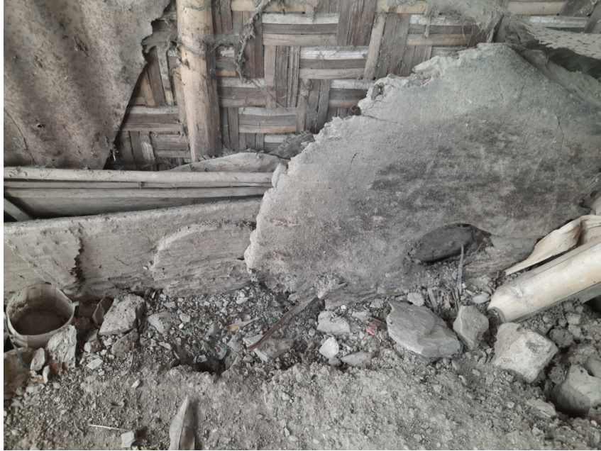
The remains of an old king post used to protect the wall from the rain water (Ighanumi Village)
