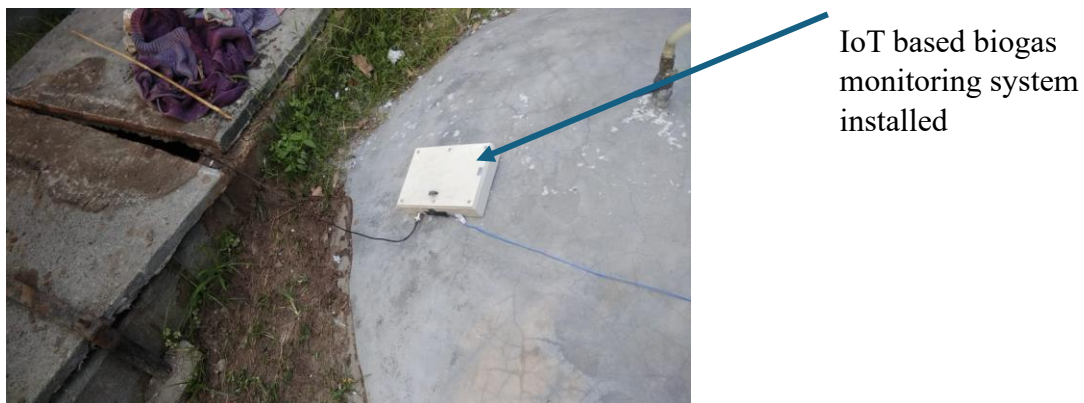
Fig 4.7 b: Installing of IoT based biogas monitoring system in 2 cubic meters Deenbandhu biogas system
