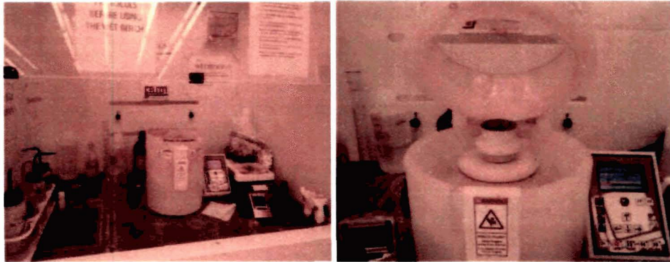
Fig-3.29: Wet Bench and Spin coater (Installed at CeNSE, IISc.)
