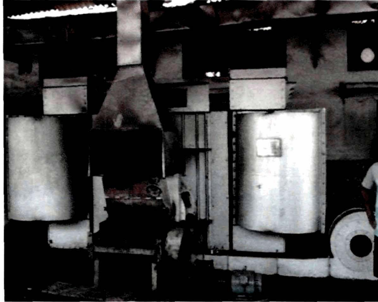
Fig.1.1 Coal fired air heater furnace
