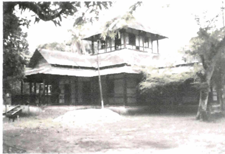
Photo 76: Residence of Late Pitambar Deva Goswami, former Satrādhikār of Garmur Satra, in dilapidated condition
