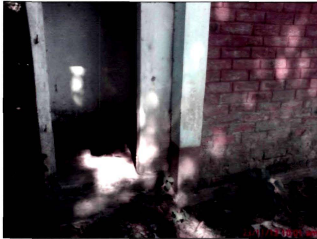
Photograph 9: Defunct toilet in a school in Noorbari Tea Garden
