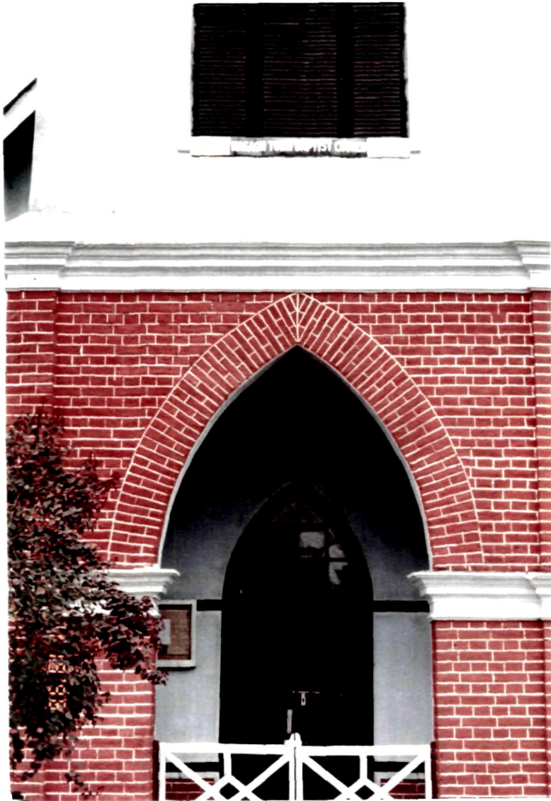
Brickwork in English bond with an arched lintel at the entrance to the Nagaon Town Baptist Church, Nagaon, Assam
