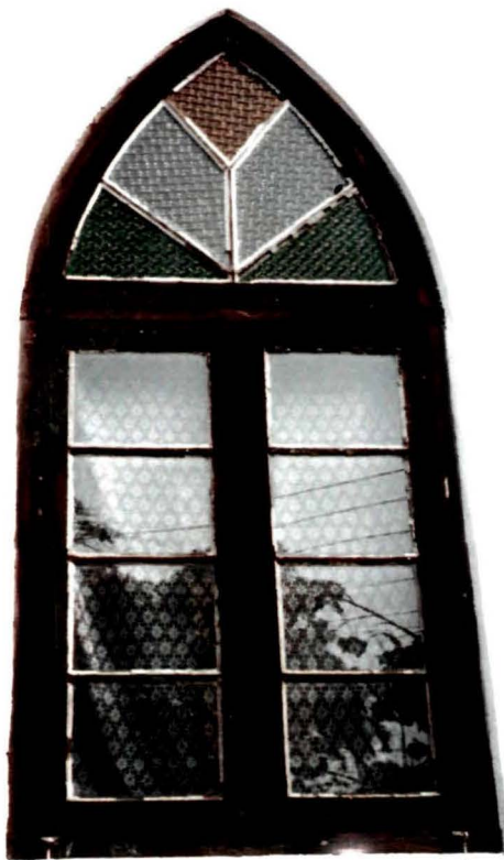
View of two windows with attached ventilators
